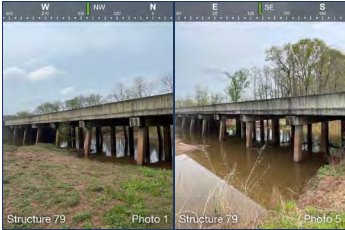
Survey photo of the bridge on the west end of the Twin Bridges Road.
