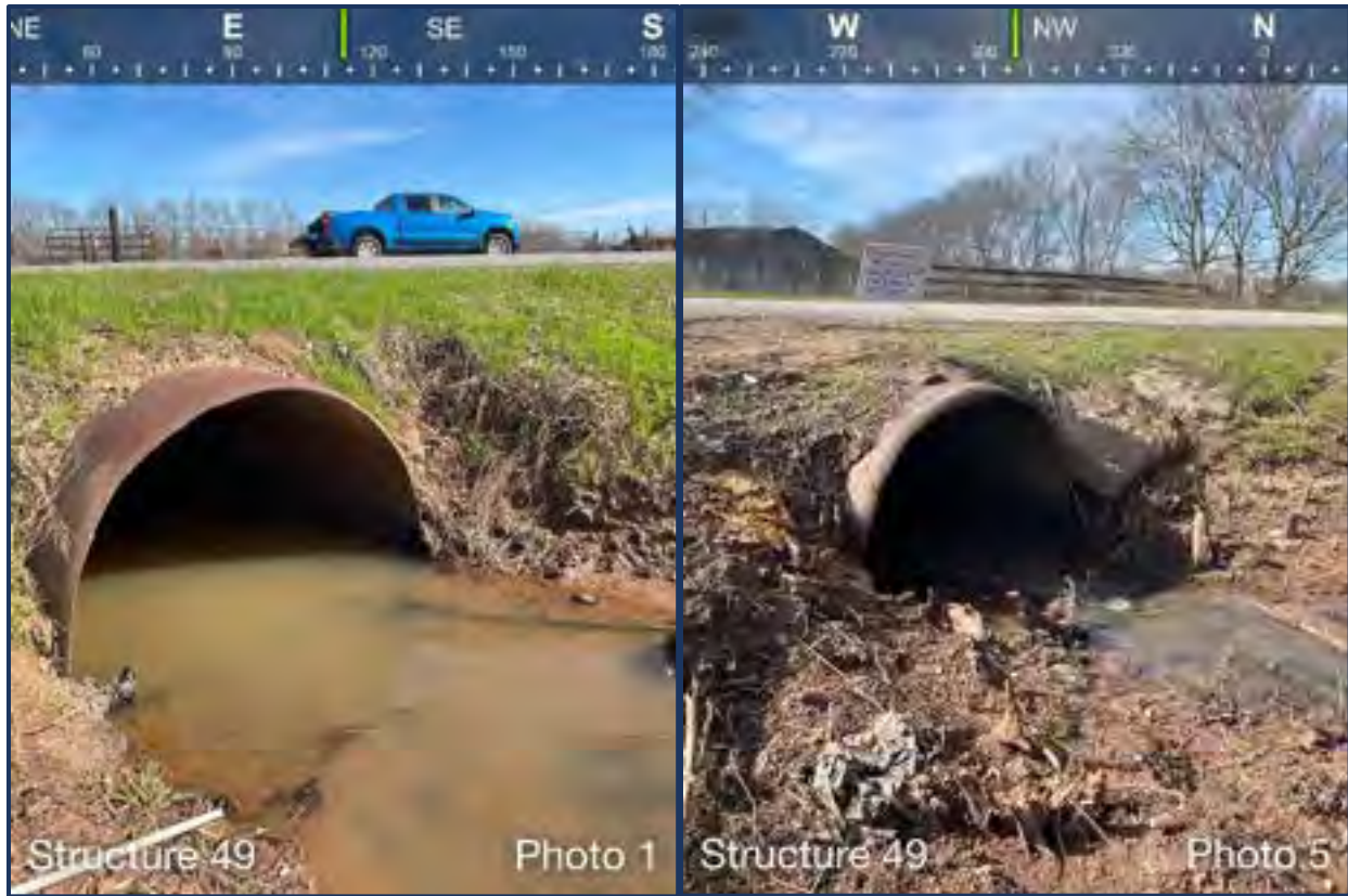
Survey photos of the culvert on the east end of the Twin Bridges Road.
