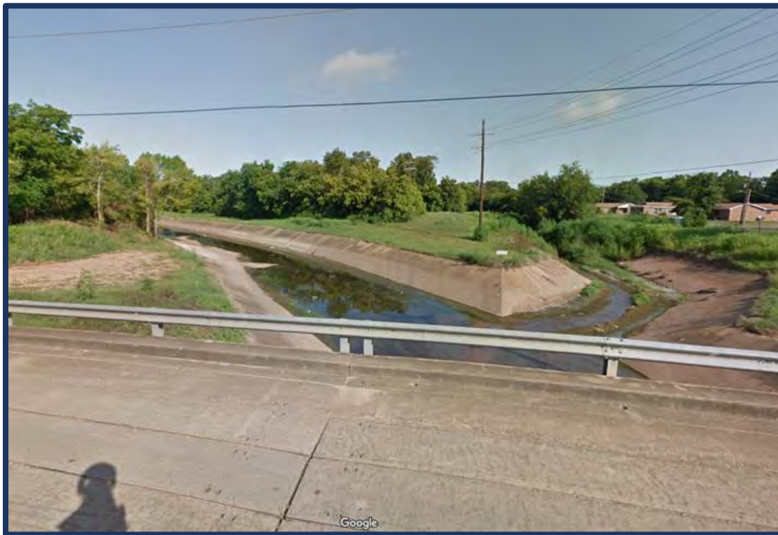
Northwest street view of the hardened portion of the Horseshoe Drainage Canal from Tulane Avenue.
